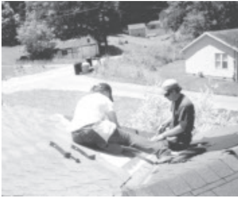
Michala Mika works hard to repair the roof of a family's home.
